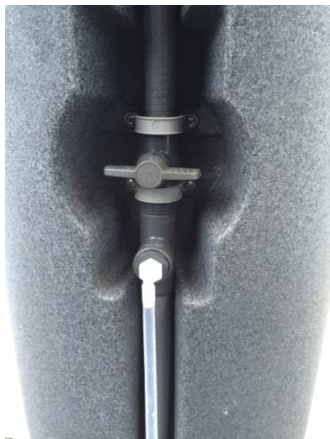
Valve in the off position
